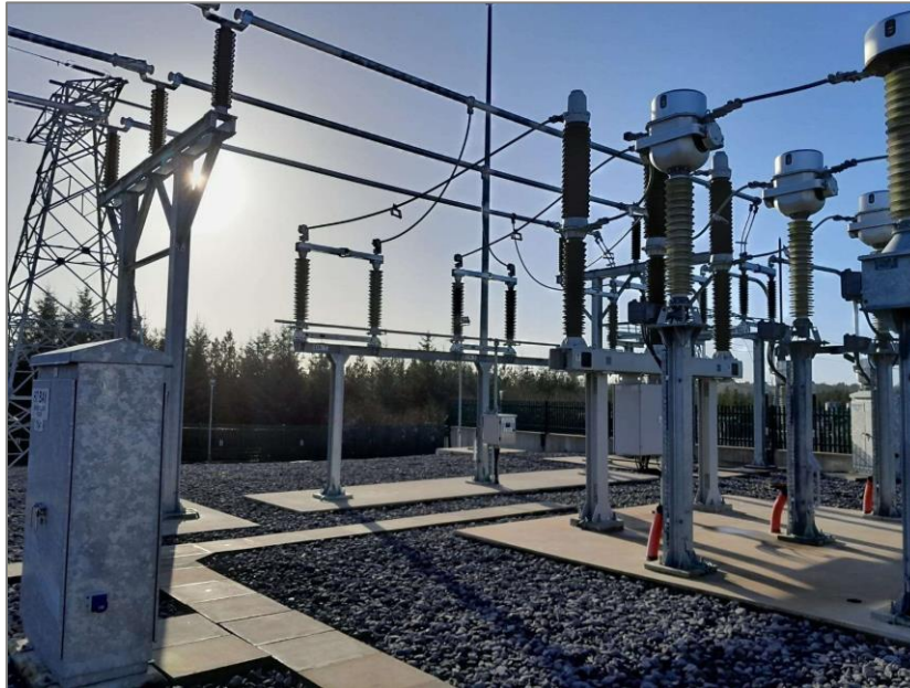
Figure 5 - Typical 110kV Electrical Infrastructure
